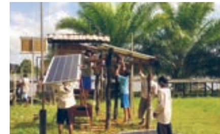
Rimba Raya funded community solar panels
